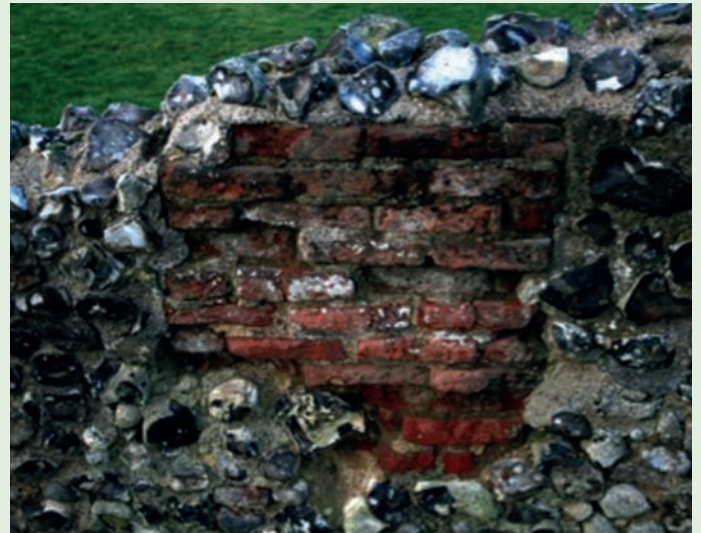
Close-up of repairs to the walls showing what is possibly Tudor brick work. Photograph: Roy Holmes.
